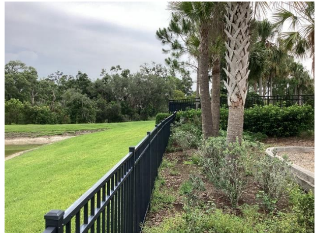
Fence leaning section
