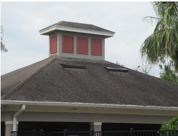
Clubhouse asphalt shingle roof (note weathering)
