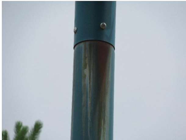
Rust at shade structure
