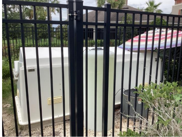
Pool mechanical equipment
