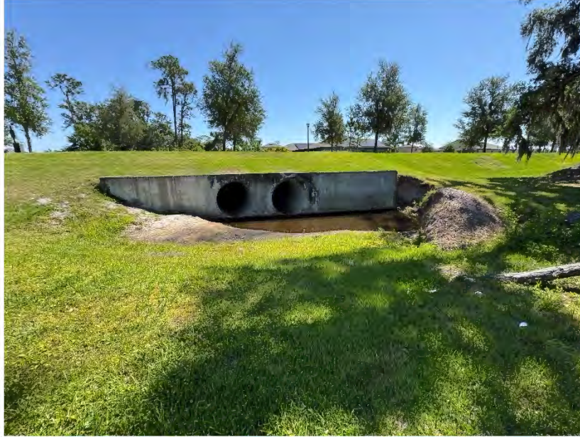
Photo 6 - Displays the erosion occurring at the dual 54 inch stormwater pipes that run under Silverado Ranch Blvd just beyond Pond H. Erosion is occurring at the right side of the retaining wall and it is recommended that District seek proposals for repair before the rainy season in May/June 2025
