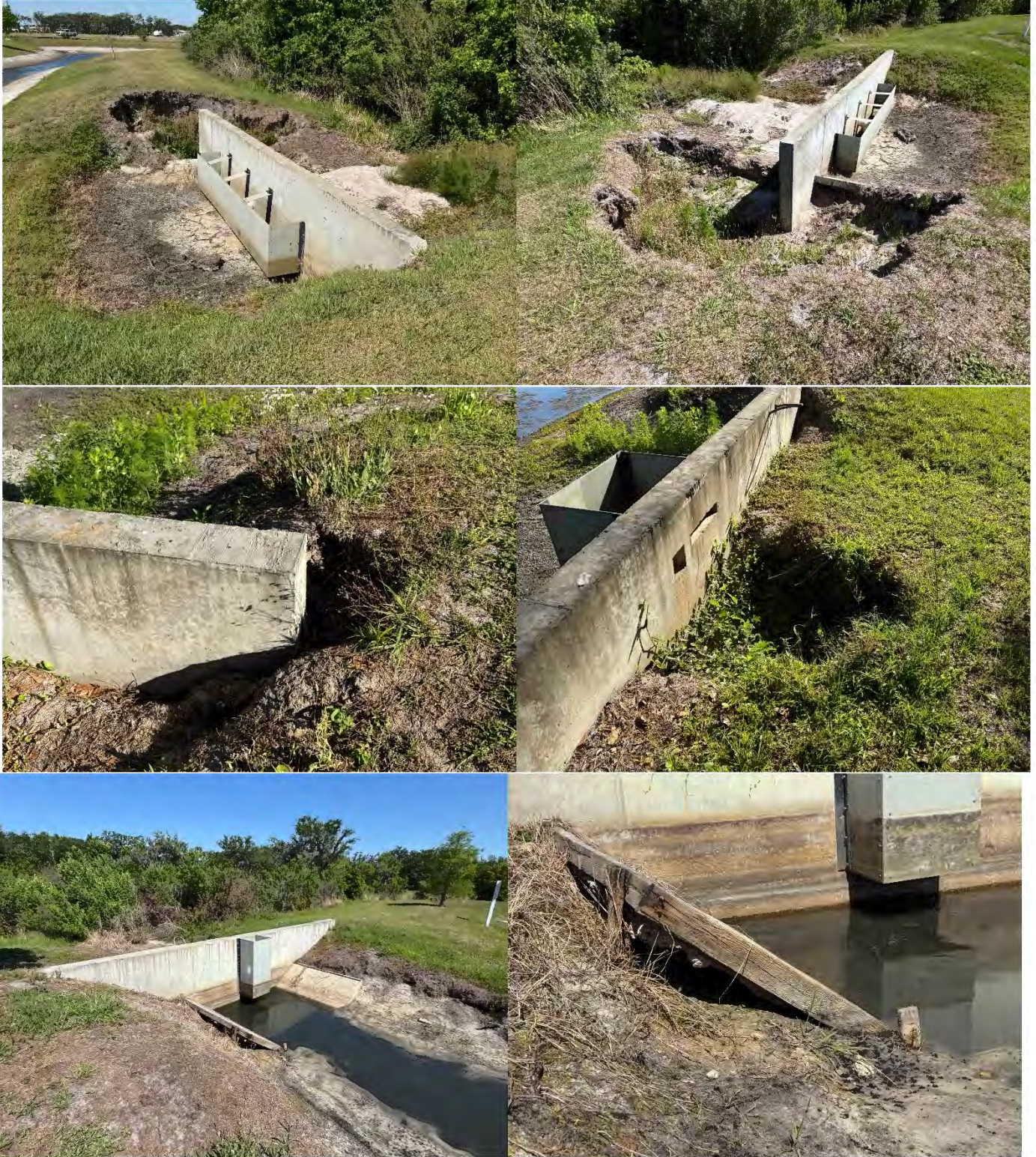
Photo 1- Displays the failed structure at Pond W2 (top), the near failed structure at Pond K (middle), and the erosion around the ditch paving at Pond W2 (bottom).
